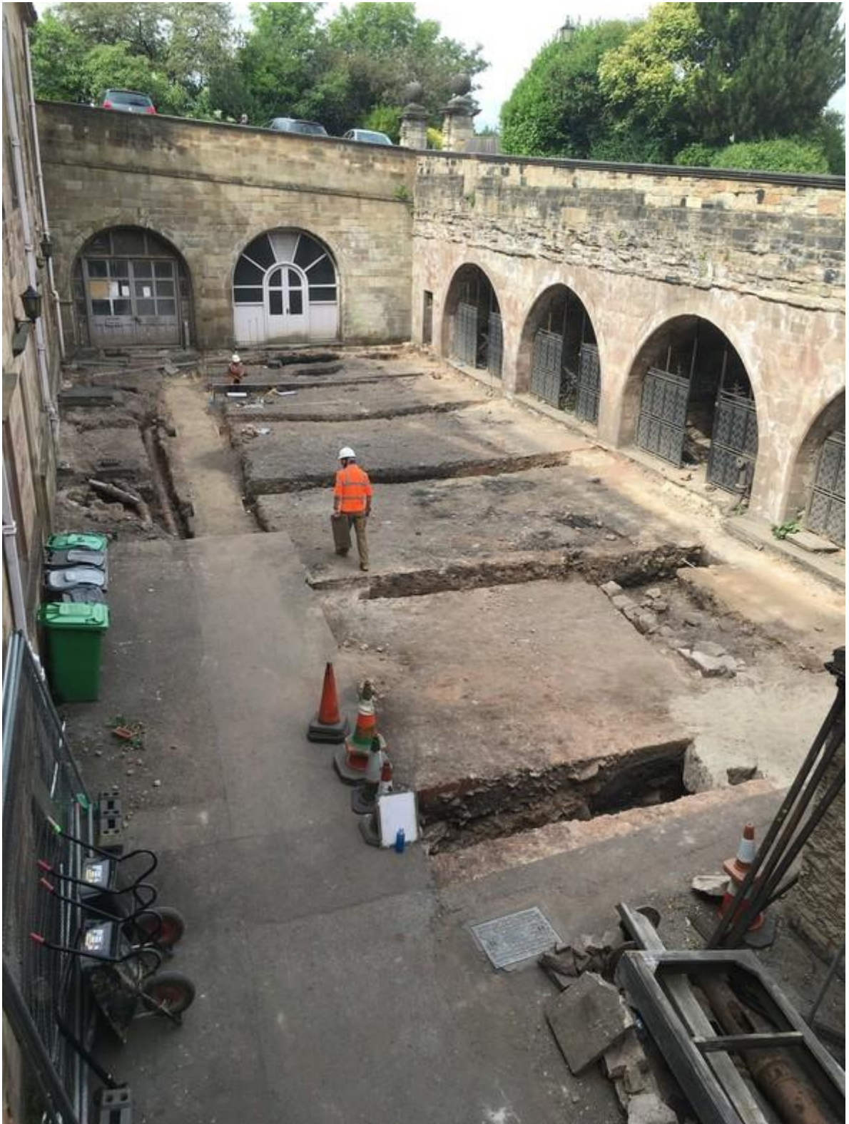
Work on the excavations on the Service Courtyard which took place last year
